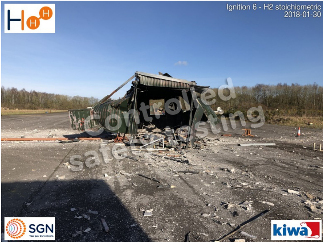
Figure 20: View of end wall of FIB after ignition 6 (100kW hydrogen) The FIB's metal doors have been torn apart from FIB frame during the explosion. Debris from inside FIB is visible on the ground outside.
