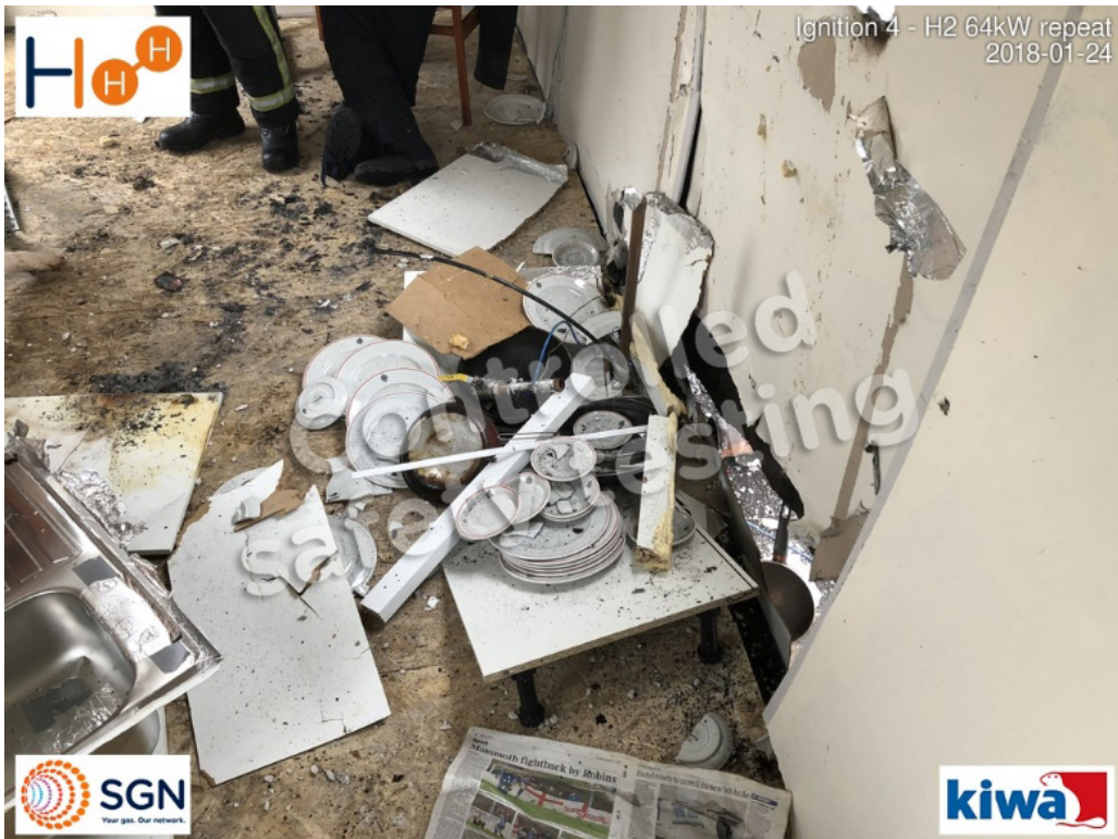
Figure 45: Close-up of damaged sink cupboard and damage to FIB wall
