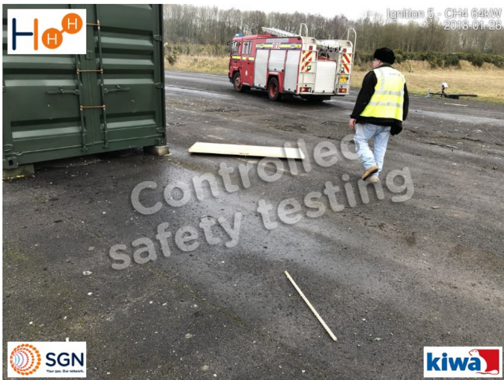
Figure 49: Blown out door and door surround (foreground)
