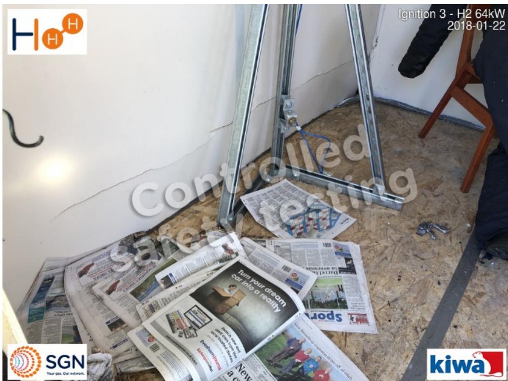
Figure 41: Damaged plasterboard at floor-level (approx. 30cm from ground and 2m long), indicating some pressure-relief was through the walls
