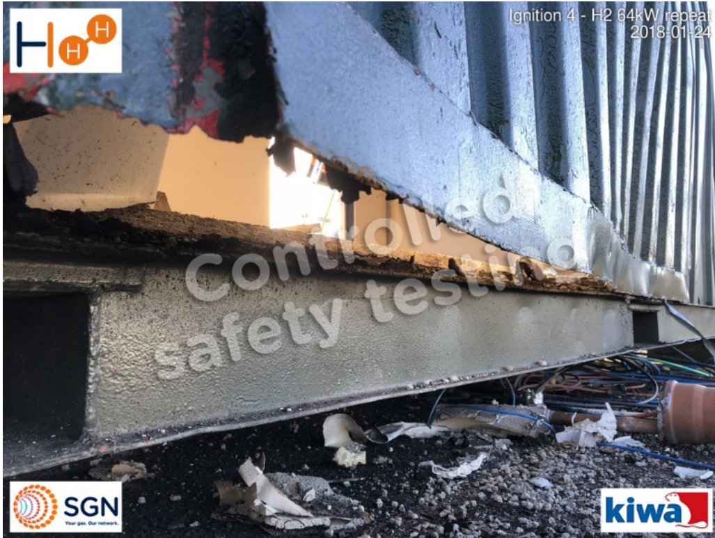
Figure 44: Close-up of damage to FIB wall showing 10-20cm gap in weld
