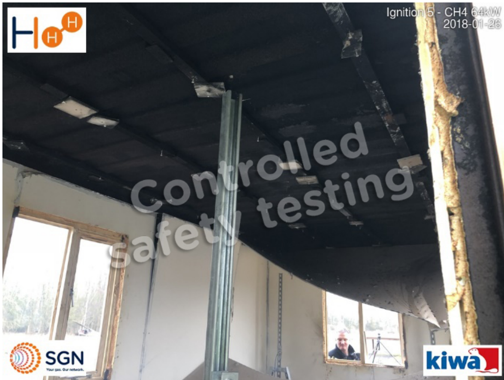
Figure 50: Internal view of FIB showing collapsed ceiling
