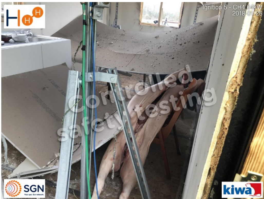
Figure 51: Collapsed ceiling in pig carcass
