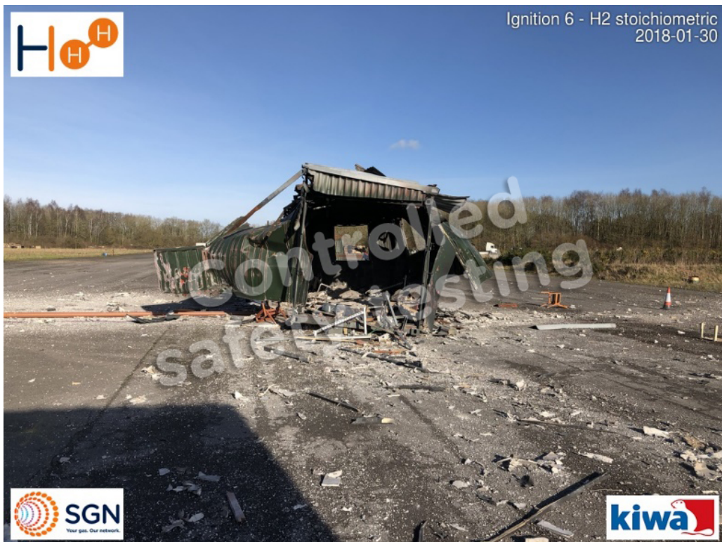
Figure 55: View of end wall of FIB (doors have been torn apart from FIB frame during explosion). Debris from inside FIB visible on the ground outside, including pressure measurement stand (centre)
