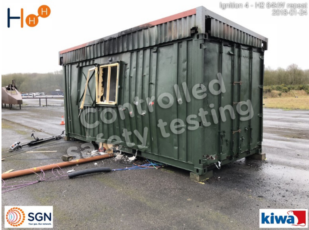
Figure 42: View of blown out sink window showing damage to FIB wall near sink cupboard
