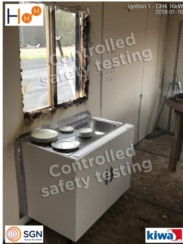
Figure 31: View of sink (undamaged) and blown out window frame
