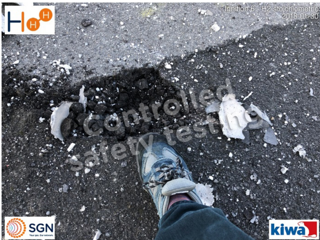
Figure 59: Damage to tarmac approx. 10m from end wall of FIB
