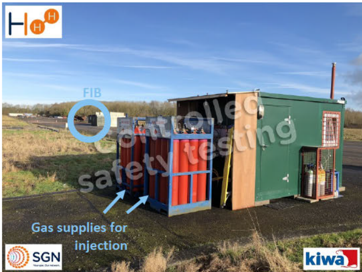
Figure 6: Control cabin and gas supplies
