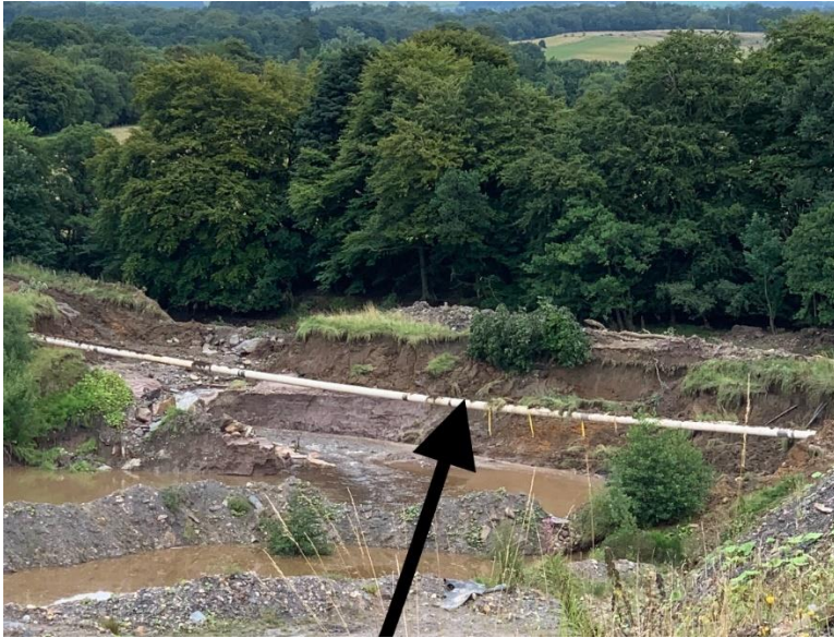
Figure 3: Pipeline washout at Forestmill, Scotland 2020
