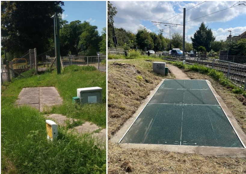
Figure 3: Gatic at Tidworth Road, Hampshire
