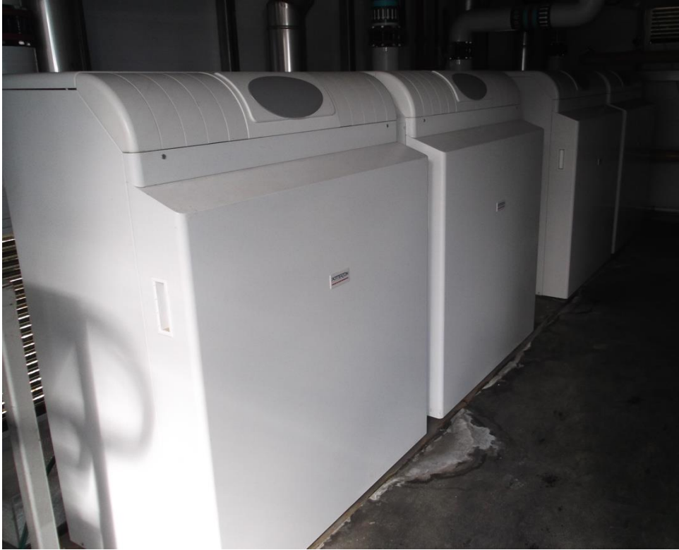
Figure 3: Boilers At Hardwick Offtake (Southern Network)
