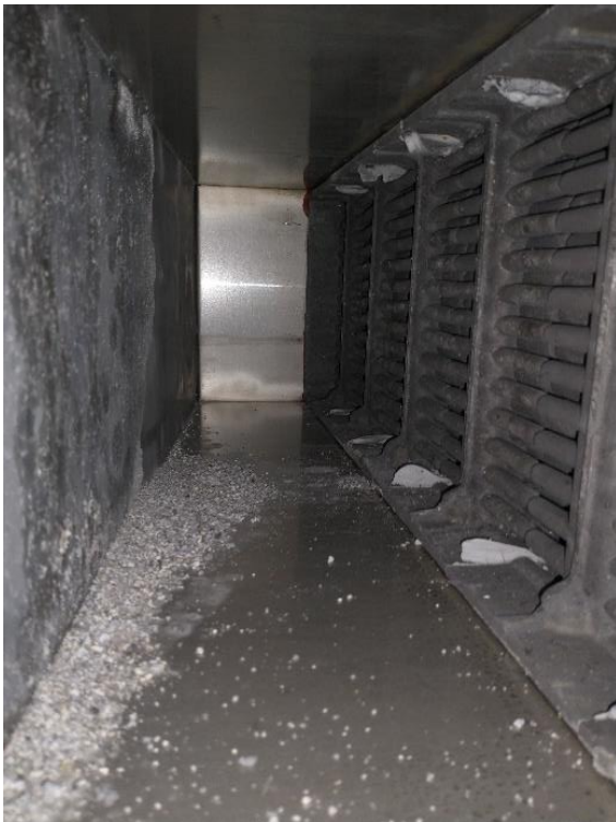
Figure 8: Image showing internal deterioration of aluminium heat exchanger.
