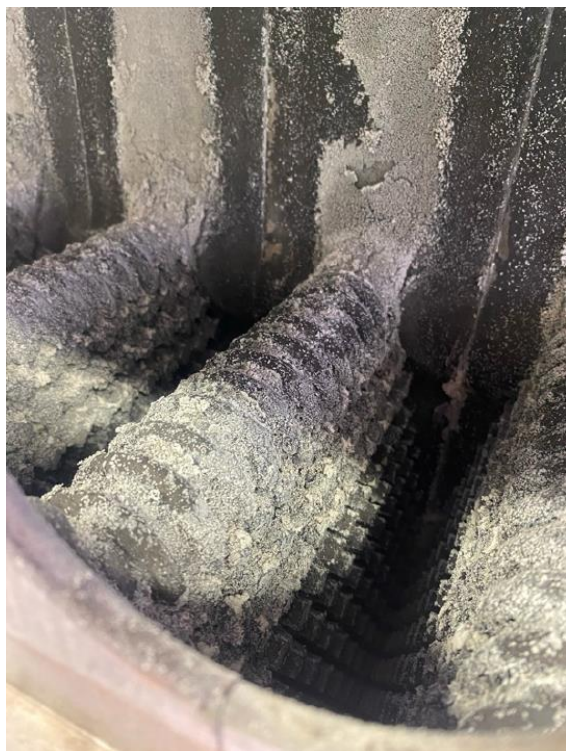
Figure 9: Image showing internal deterioration of aluminium heat exchanger.
