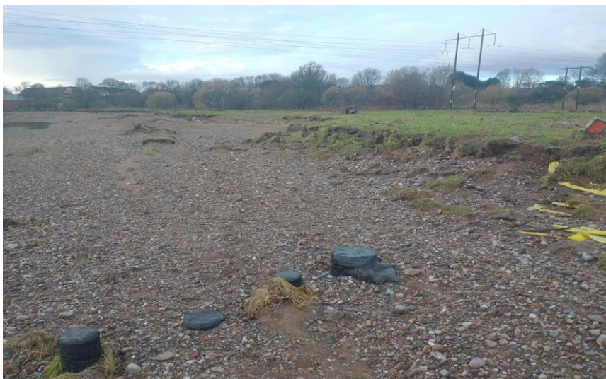
Figure 5: Flood plain soil erosion and exposed Intermediate Pressure (IP) pipe fittings
